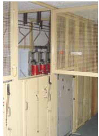
Transformatorstation Hofwies, Ehrendingen
